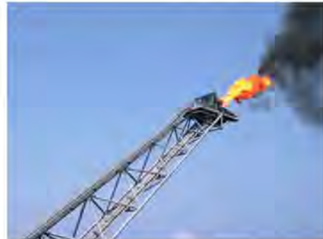
Darflare™ heat shield installed on the Chevron Benchamas platform, Thailand.
